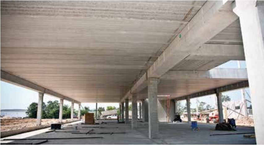
The total-precast concrete structural system provided open 40-foot bays that allowed flexibility in laying out offices. Photo: Kerkstra Precast.
